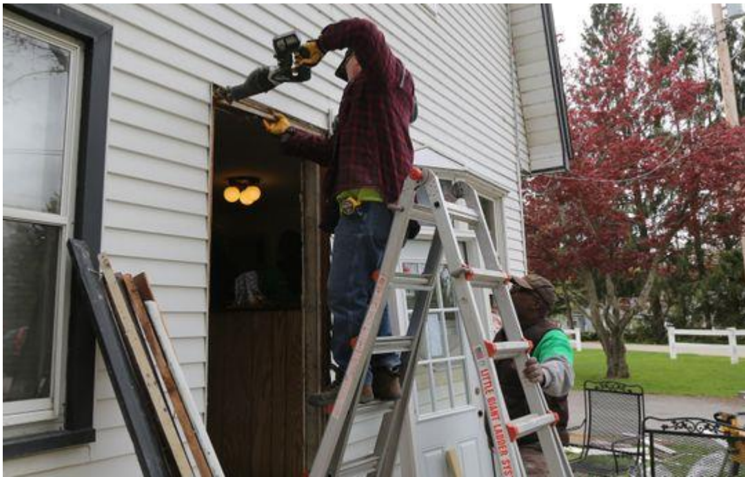
Marc Dennis (right), of Beacon, holds the ladder for Larry Theisen, of Hyde Park, as he works on replacing the front door of Lee Baker's Hillside Lake home. The volunteers were two of 25 who were working on the home. (Photo: Jack Howland/Poughkeepsie Journal)
